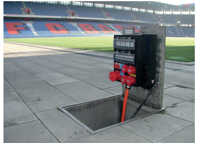
Underfloor distributor system, St. Jakob-Park stadium in Basel
